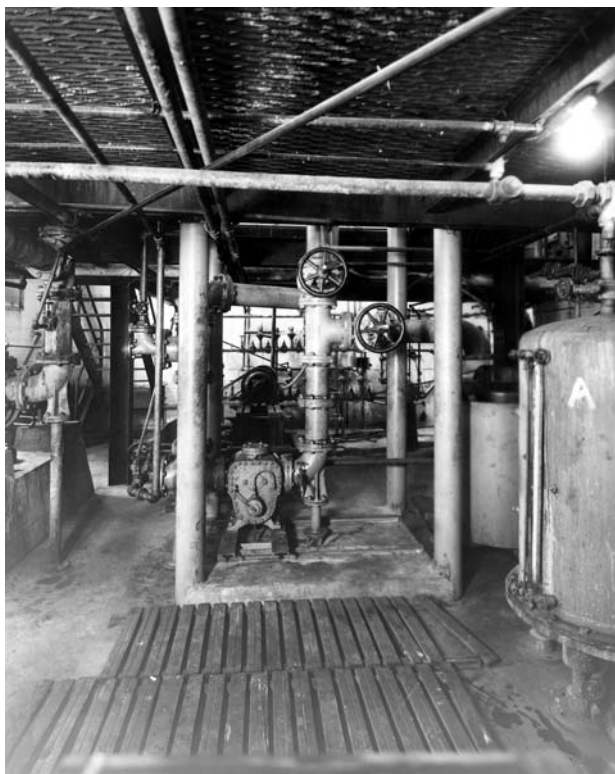
Basement of the high-bay area in the East Engineering evaporator laboratory during the student days of Drake Parker. “A” is a drip tank for measuring condensate, and there is a vacuum pump in the left center.
